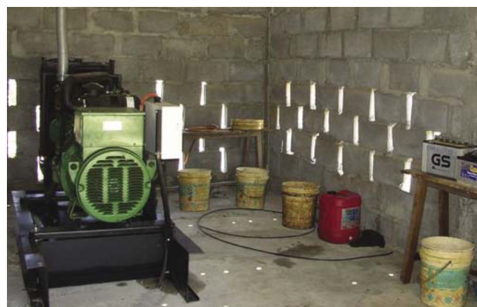
The new diesel generator funded by USAid
